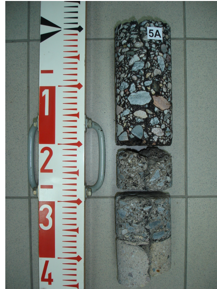
Figure 2. A specimen cored out at the crack in the national road No. 7. The crack propagates through the entire pavement.
