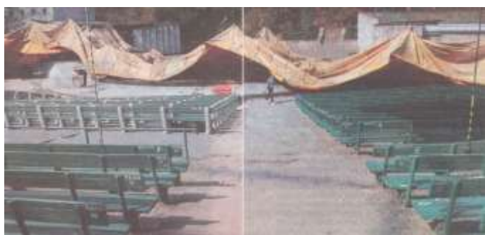
Figure 1. Putting down the roofing structure of the Forest Opera in Sopot (Poland) before winter season (Dziennik Bałtycki 2007).
