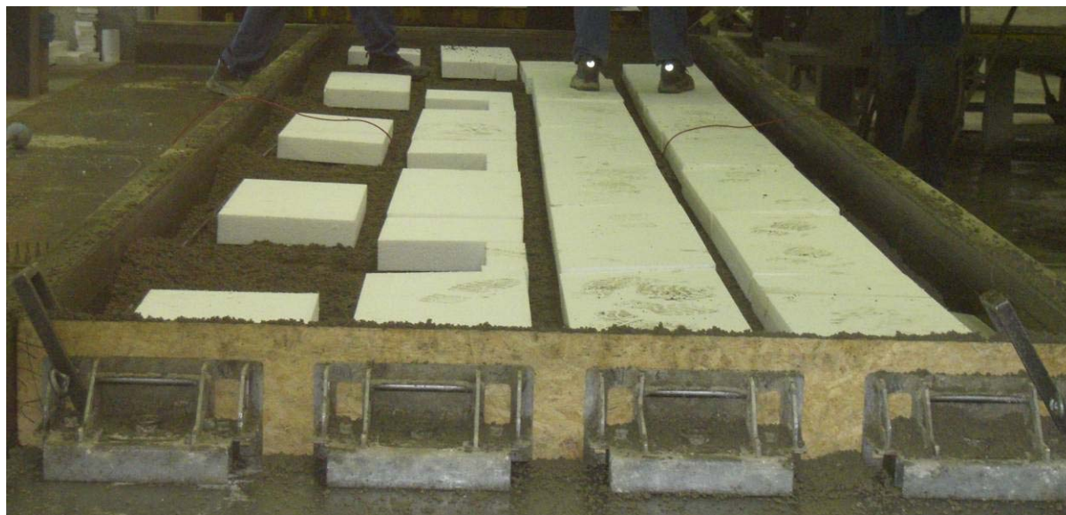
Figure 3. The reinforced wall component (the first improved type) during the concreting process
