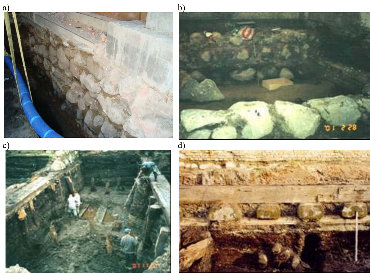
Figure 1. Foundations: a) a historical building in Olsztyn in Staromiejska Street, b) a Romanesque church in the Market Hall in Gdańsk, c) old granaries in Basztowa Street in Gdańsk, d) old granaries in Chmielna Street in Gdańsk
