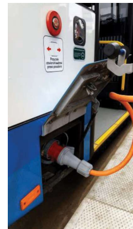
Fig. 10 Charging of traction batteries from 400 VAC grid on a terminus
