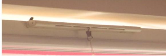
Fig. 2. Typical inlet gaps in Poland
