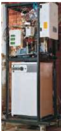
Fig. 8. General view of the micro-CHP ORC unit.
