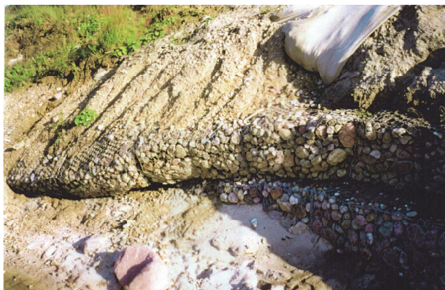
Fig. 3. Gabions composing the seawall in the region of "Bałtyk", damaged in 1998 (photo courtesy of W. Subotowicz)
