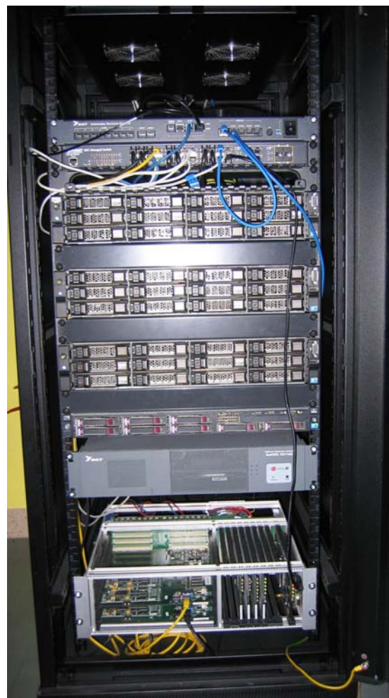
Figure 2. From the top: URC for OP, switch, Archive Servers (AS), voice recorder, telephone server.
