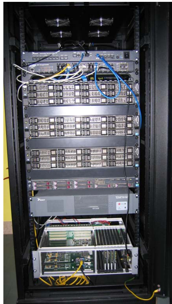
Figure 2. From the top: URC for OP, switch, Archive Servers (AS), voice recorder, telephone server.
