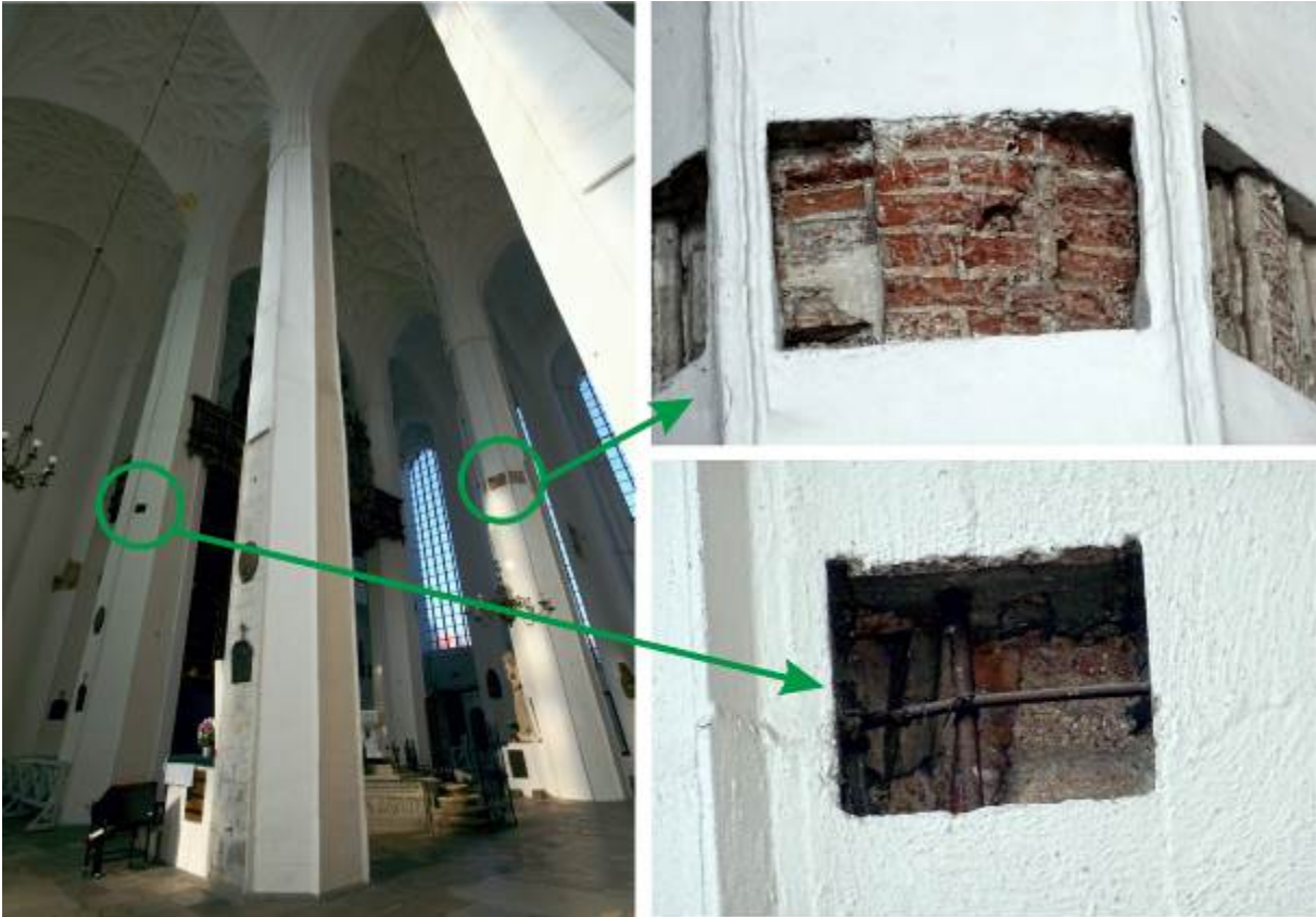
Figure 5. Plastered pillars with open areas showing details of masonry and reinforced masonry
