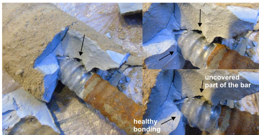
Figure 7.31 Damaged anchor: uncovered part of the bar and healthy connection at the anchorage place
