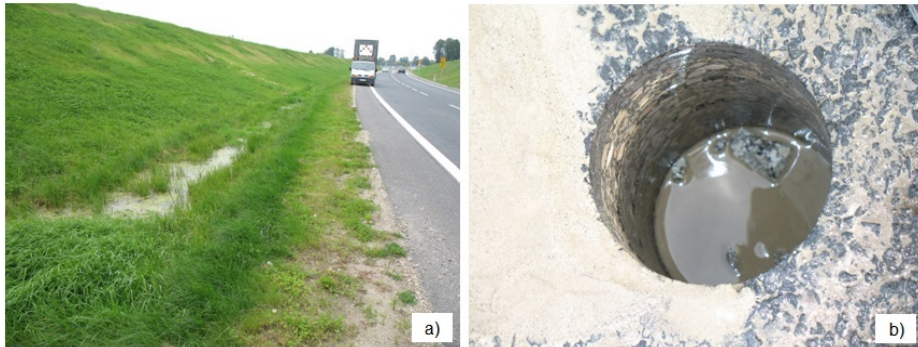
Fig. 3. a) section of road on which the drainage system is not functional; b) core extraction spot cleaned of dirt and water, spontaneously filling with water coming up from below.
