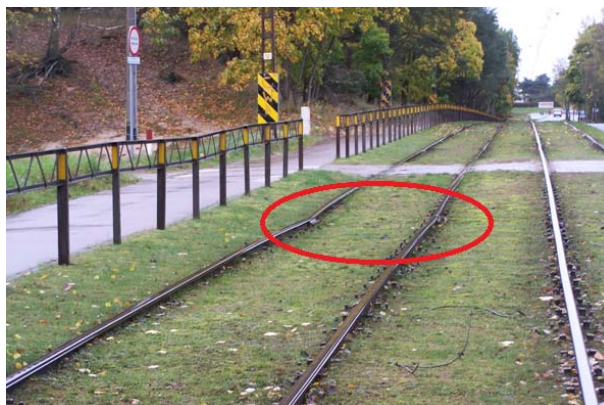
Fig. 3. Displacements of the sleepers in the track
