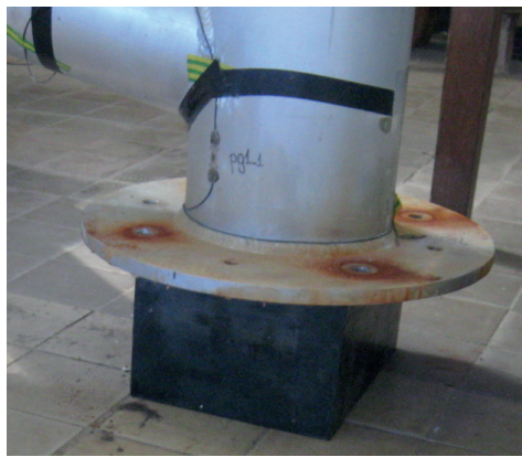
Fig. 2. Conditions of tripod foundation on rubber blocks.
