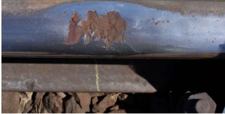
Fig. 1. Squat-type rail defect.
