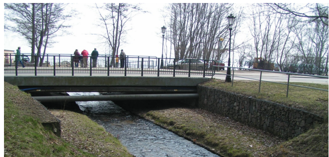
Fig. 4. The bridge over Kacza river in line of Orłowska street in Gdynia (a photo from this author's archive),
