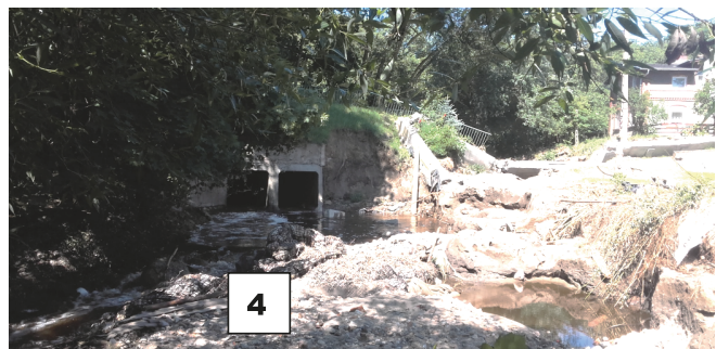
Fig. 2. Damages in the Kacza river estuary area in Gdynia Orłowo as a result of the freshet in July 2016 (photos No. 1, 2, 3 – washout of sea-shore belt below Orłowska street bridge, photo No. 4 - breach in road embankment of Zapotoczna street. Location of subsequent shots – see Fig. 1. ( acc. this author's archive)
