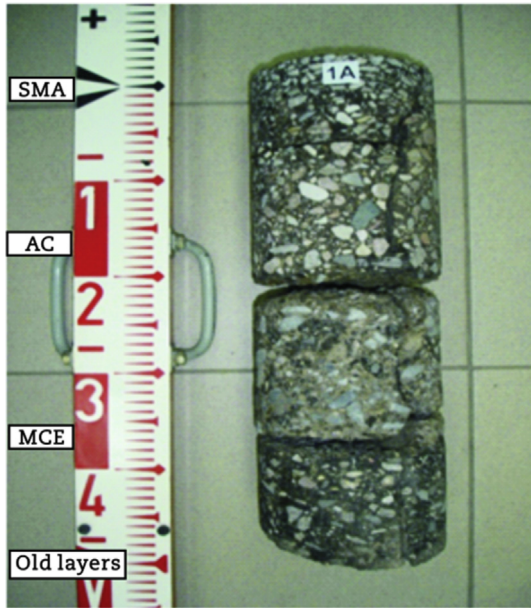
Fig. 6 – Crack propagating through asphalt courses and an MCE base.
