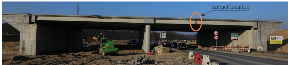
Fig. 1 General view of the bridge and the location of the impacts.
