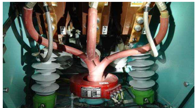
Fig. 4. Capacitive couplers installed at point A.
