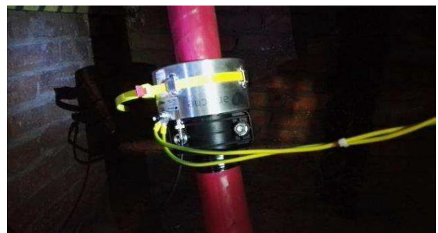
Fig. 5. Inductive couplers installed at point A.
