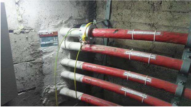
Fig. 6. Inductive couplers installed at point B.
