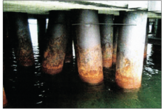
Fig. 6. Sea corrosion of piles [10]
