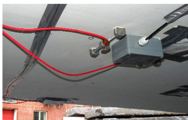
Figure 7. VWSG sensor fixed to the bridge.
