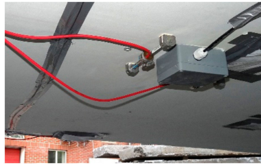
Figure 7. VWSG sensor fixed to the bridge.
