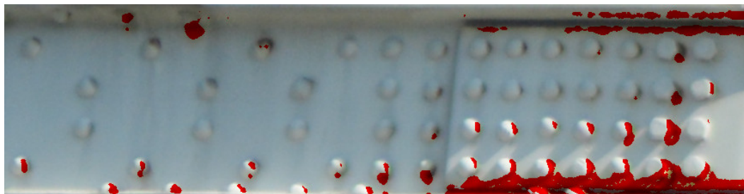
Figure 16. Rust detection: (A–B) close-up to nodes and (C) close-up to rivets.
