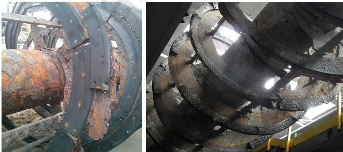
Photo 4÷5. Classifier's spirals degraded due to corrosion.
