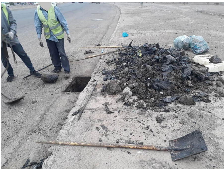
Fig. 11b. Municipality workers cleaning an inlet, which was almost completely filled with waste
