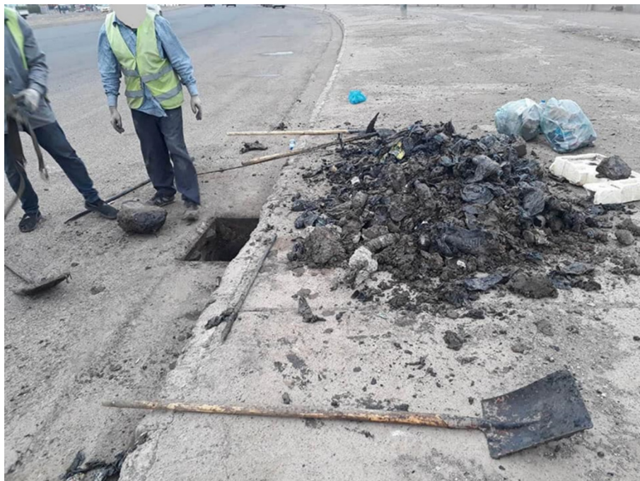
Fig. 11b. Municipality workers cleaning an inlet, which was almost completely filled with waste
