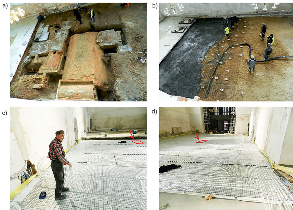
Fig. 1. Photograph of the floor in St. Joseph's Church in Gdańsk, Poland (Google Maps coordinates in a WGS84 system: 54.354111 N, 18.647135 E): a) excavation view, b) concreting of the reinforced concrete slab, c), d) floor heating view with marked locations of the entrances to the crypts.
