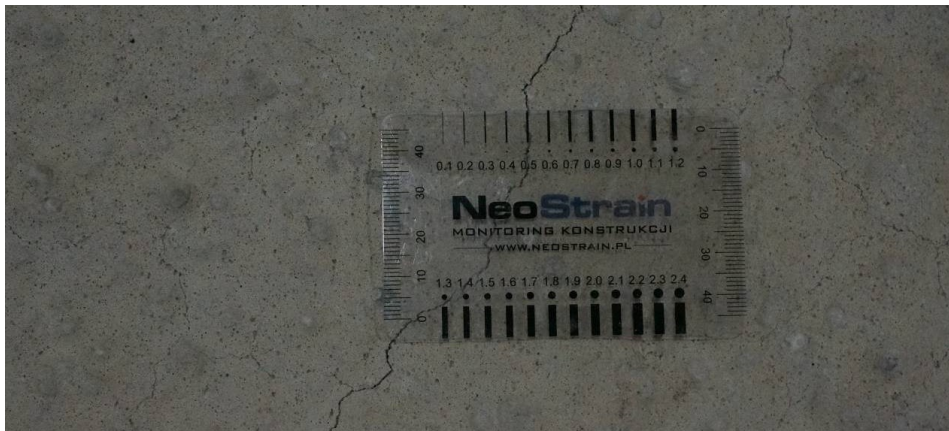
Fig. 10. Measurement of the cracks in sample no. 4.
