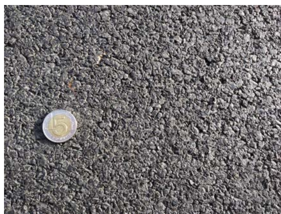
Figure 20. Close-up view of the poroelastic wearing course.
