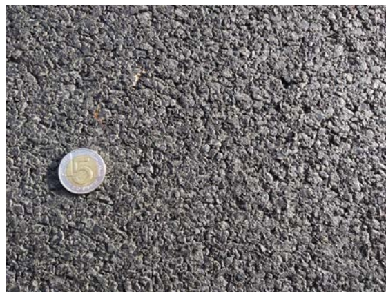
Figure 20. Close-up view of the poroelastic wearing course.
