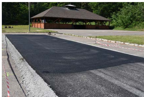
Figure 14. Binder course AC 16W before installation of different types of wearing courses.
