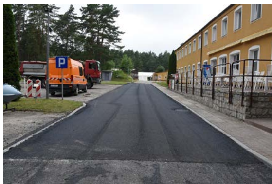
Figure 21. Longitudinal marks caused by paver screed joints on the Dąbrówka trial section.
