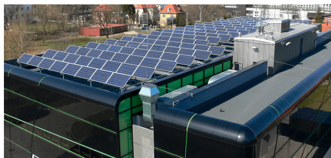
Figure 5. A view of photovoltaic panels installed on the roof of the LINTE 2 laboratory [41].
