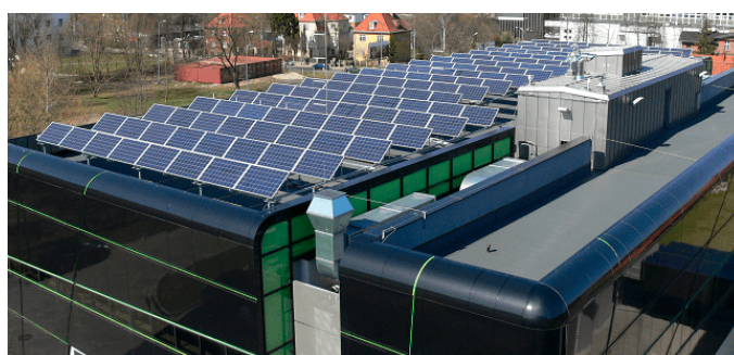
Figure 5. A view of photovoltaic panels installed on the roof of the LINTE 2 laboratory [41].
