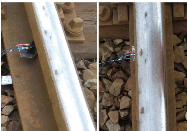
Fig. 3. Defect 221 – damage of the running surface on railway line no. 213 Reda – Hel [authors' own work]
