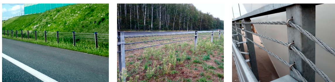
Figure 2. Examples of safety barriers using 3 \times 7 19-mm wire rope.
