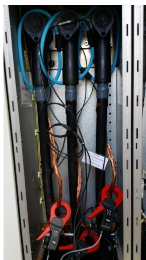
Figure 5. Measurement of currents flowing in cores and sheaths in Substation 2.
