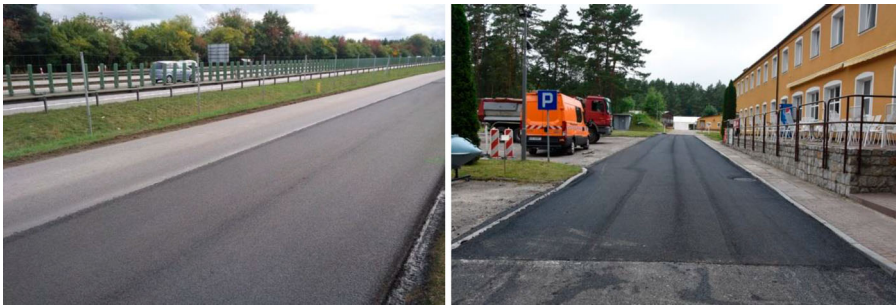
Figure 14. Longitudinal marks caused by paver screed joints on the test sections.
