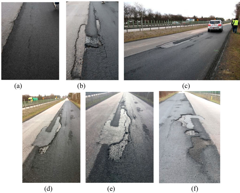
Figure 18. Deterioration of the sixth subsection of the test Section 2: (a) 22 November 2019 (51st day); (b) 13 January 2020 (103rd day); (c) 5 February 2020 (126th day); (d) 19 February 2020 (140th day); (e) 4 March 2020 (154th day); (f) 10 March 2020 (160th day).
