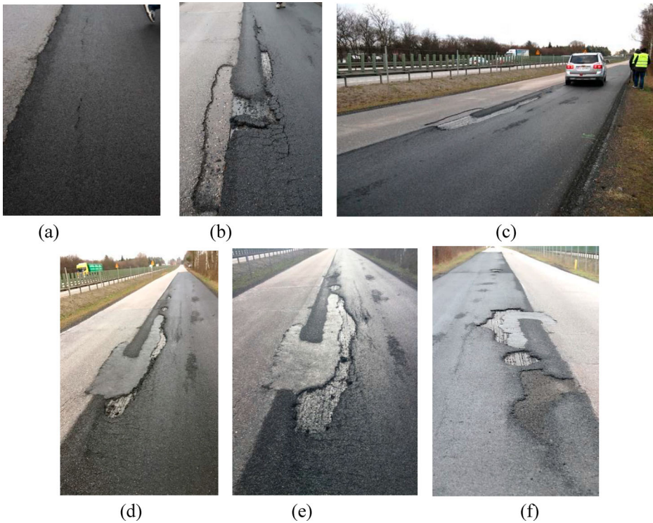
Figure 18. Deterioration of the sixth subsection of the test Section 2: (a) 22 November 2019 (51st day); (b) 13 January 2020 (103rd day); (c) 5 February 2020 (126th day); (d) 19 February 2020 (140th day); (e) 4 March 2020 (154th day); (f) 10 March 2020 (160th day).
