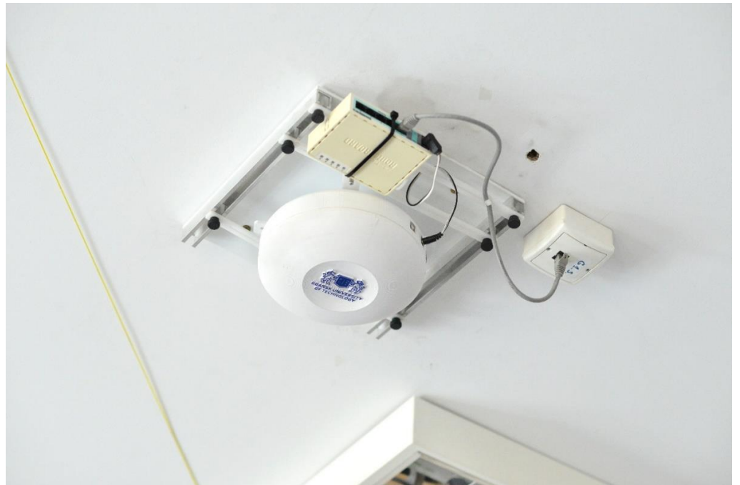
Figure 8. The ESPAR antenna integrated together with the custom-made WSN board installed within a custom-made housing and mounted on the ceiling.
