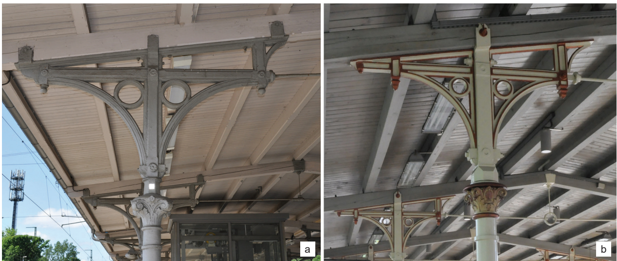
Fig. 4. Comparison of the upper parts of cast-iron columns supporting platform shelters: a) Berlin S Wannsee Bahnhof, 2019, b) Sopot, 2020 (photo by M. Kwasek)
