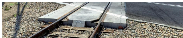
Fig. 8. Concrete level crossing slabs
