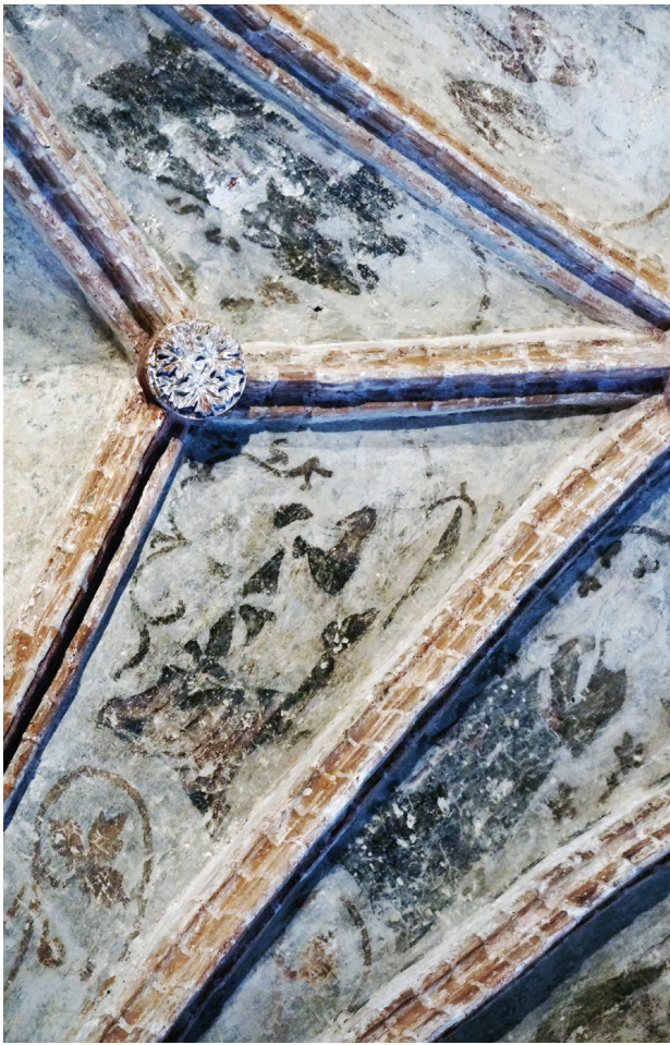
Fig. 9. Part of the northern bay vault with traces of exposed polychrome (2 nd quarter of the 15 th century?) (photo by A. Piwek)
