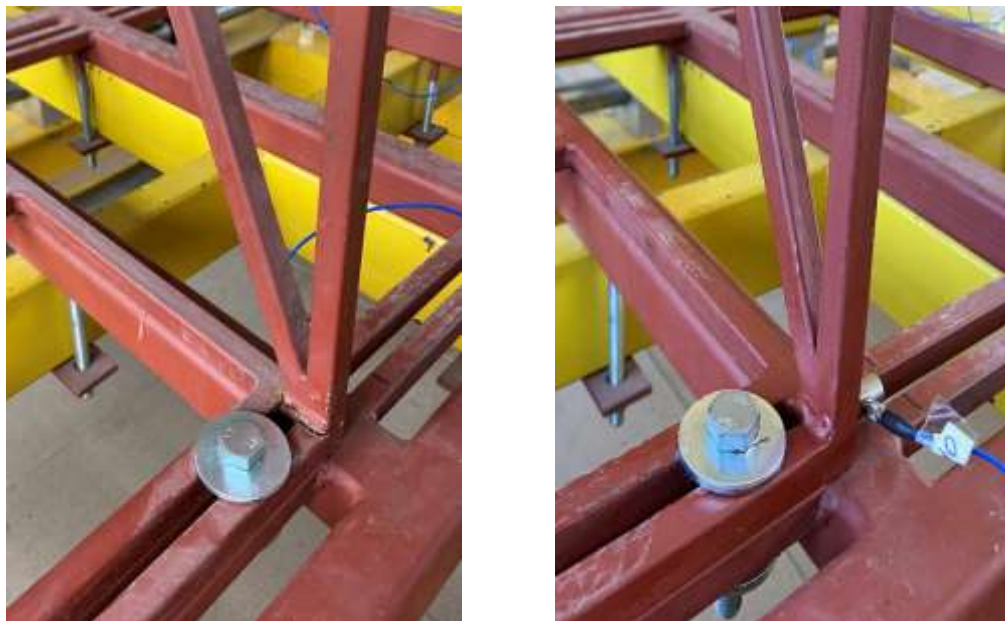
a) Destroyed joint
