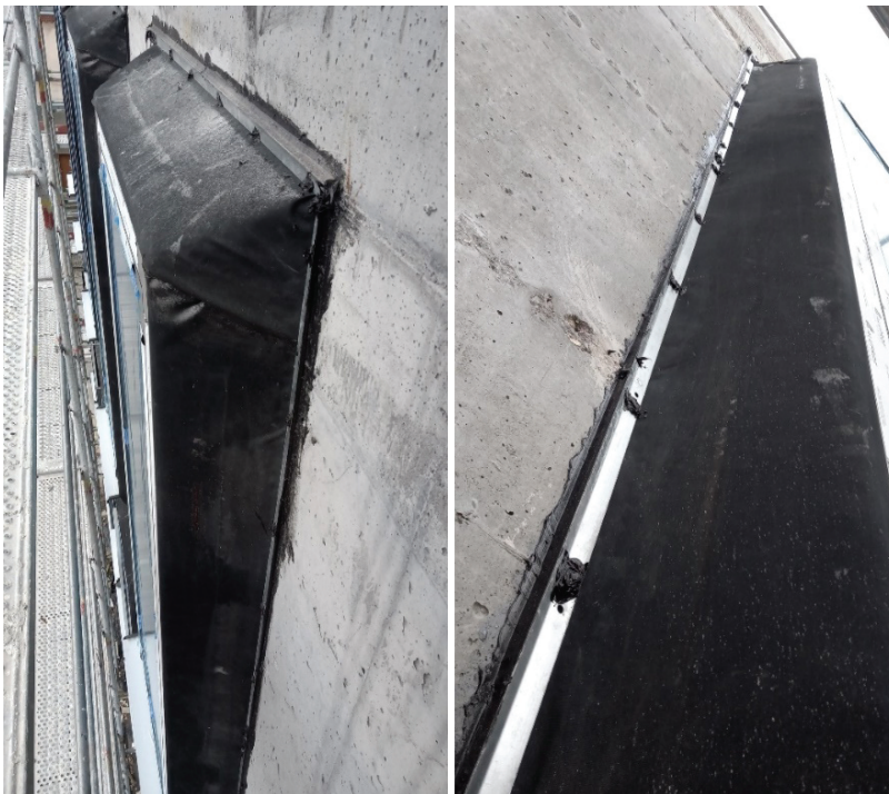
Fig. 1. Outside apron EPDM membrane in a window façade system fastened to reinforced concrete wall
