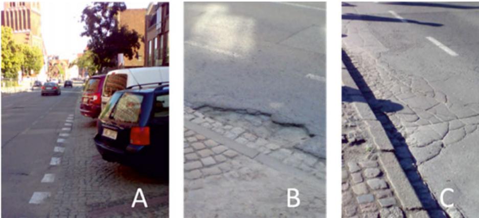
Fig. 2. Cycle lane Rajska–Podmłyńska: a) side parking b) uneven surface c) cracked surface
