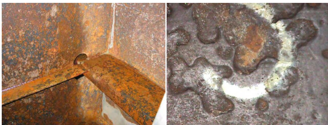
Figure 1. The comparison between general (left) and pitting (right) corrosion (International Association of Classification Societies, 2015).
