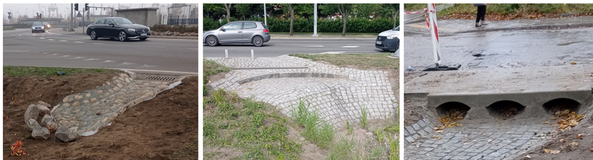
Fig. 5. Existing inlets examples from rain gardens in Gdańsk (photo M. Kasprzyk).
