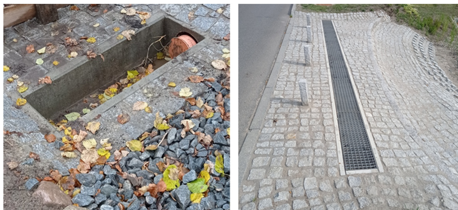
Fig. 6. Examples of settling tank installations (photo M. Kasprzyk).
