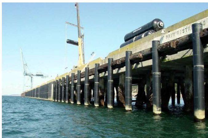
Fig. 2. CFFT piles protecting the wharf from ships mooring at the Hadlock military port on Indian Island, Washington, USA [6], [9]
