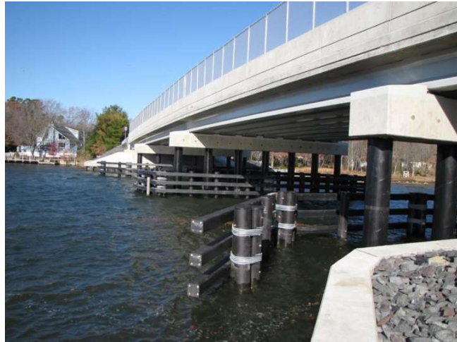
Fig. 4. CFFT piles protecting the intermediate supports of the bridge in Lacey Township, NJ, USA [7]
