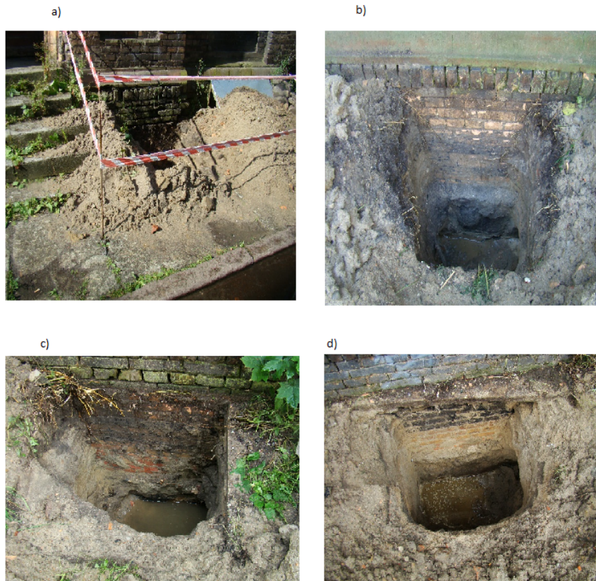
Figure 5. Building planned for modernization - outcrops from the side of the elevation: a) north-east, b) north-west, c) south-west, d) south-east
