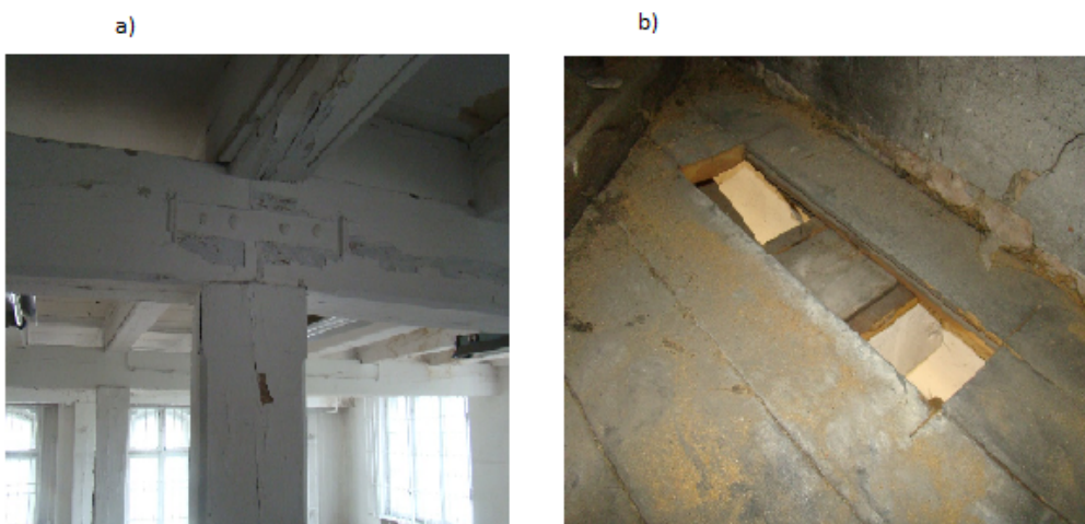
Figure 9. Building planned for modernization - ceiling above the second floor: a) a fragment of a wooden frame, b) a structure of the ceiling
