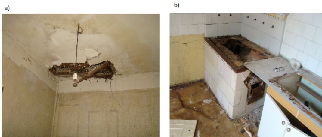
Figure 12. Building planned for modernization – lokale mieszkalne: a) broken ceiling above the ground floor, b) depreciation of equipment
