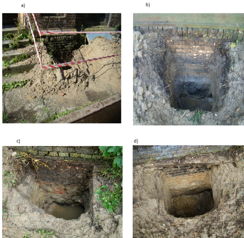
Figure 5. Building planned for modernization - outcrops from the side of the elevation: a) north-east, b) north-west, c) south-west, d) south-east
