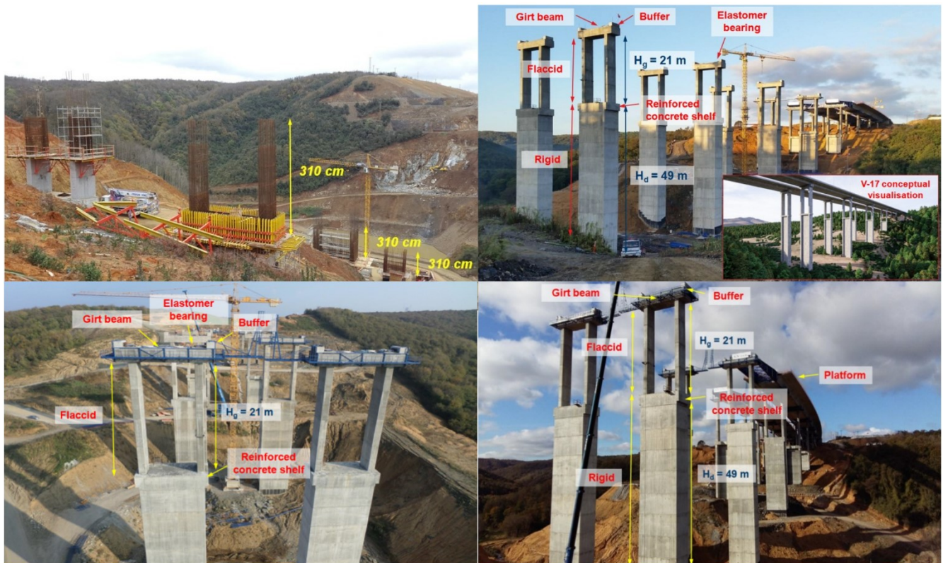
Figure 5: Photos from the implementation of the new DDC2 algorithm on the Northern Marmara Highway construction site
