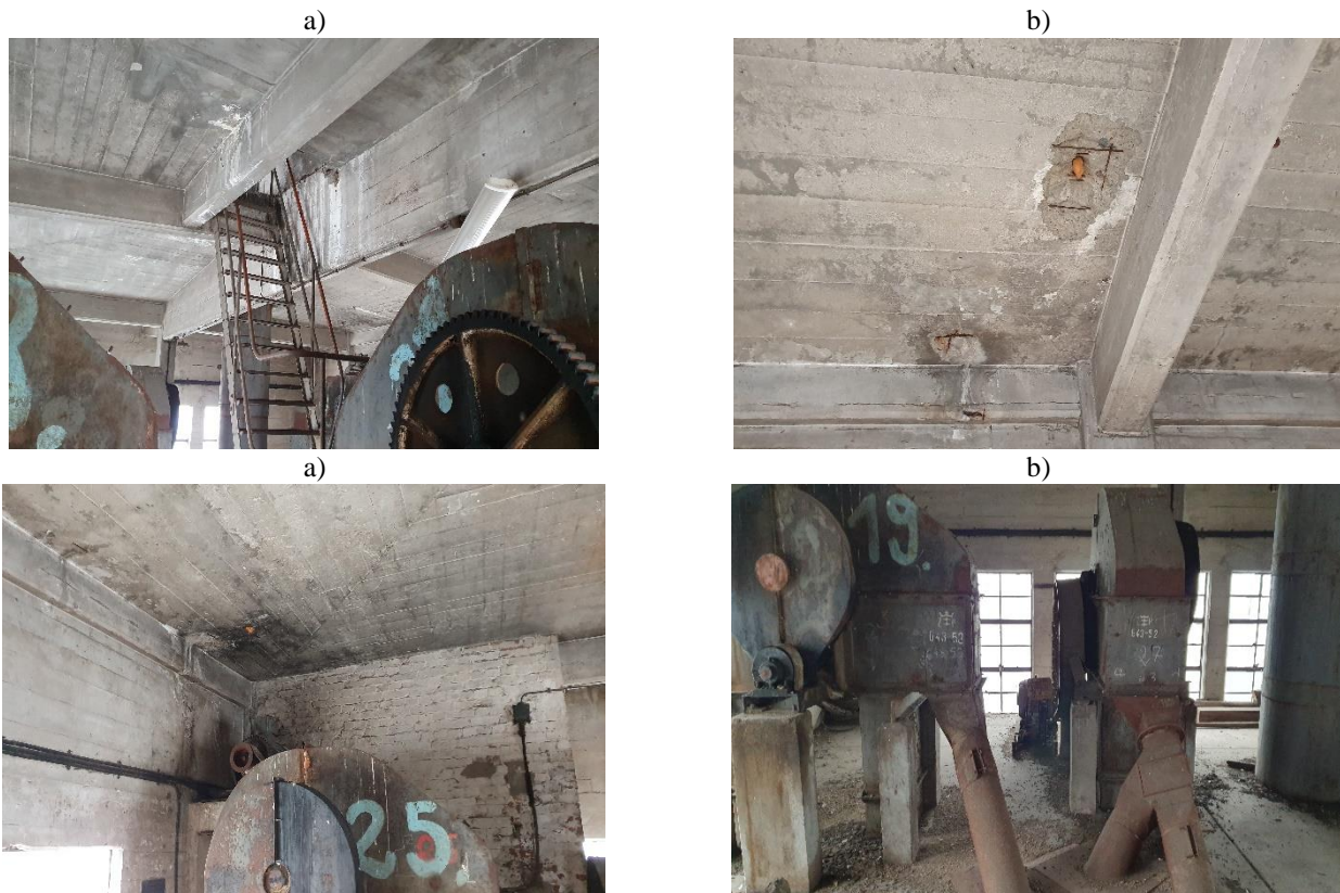
Photo 3: Grain Elevator building - level +10: a) mechanical damage to structural elements, b) defective and incomplete equipment for transporting loose materials
