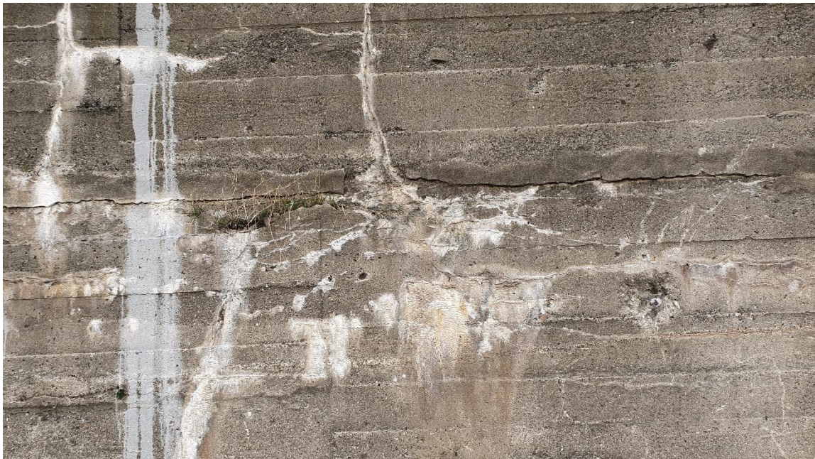
Photo 2: Examples of calcium carbonate leaks on the south-west elevation (external gable (transverse) wall from the land side (left)) of the Bunker building
