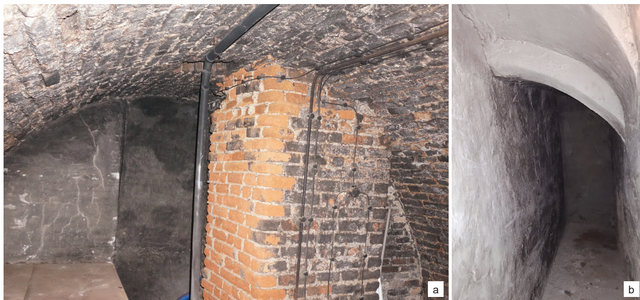
Fig. 6. Underground parts connected with the chapel at St. Joseph's Church in Gdańsk: a) a view of the interior of the crypt under the eastern part of the chapel towards the south, b) a fragment of the present corridor connecting the former crypt with the chancel (photo by A. Piwek)
