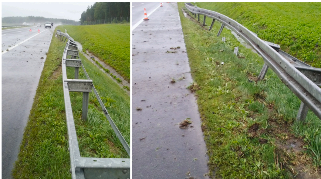
Fig. 12. General view of the accident no 2, source of photo: GDDKiA, Poland.
