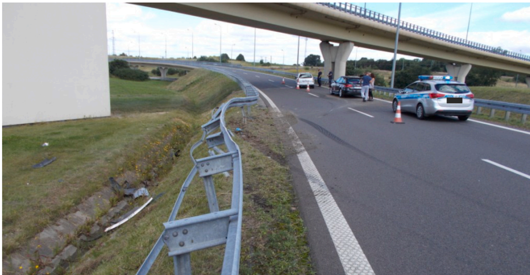
Fig. 9. General view of the accident no 1, source of photo: GDDKiA, Poland.
