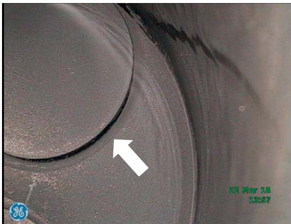
e) Bottom plate of the cylinder head – ajar outlet valve, closed inlet valve
