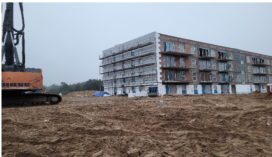
Figure 6: The examined case: vibration-resistant structure located near the soldier pile wall realization.
